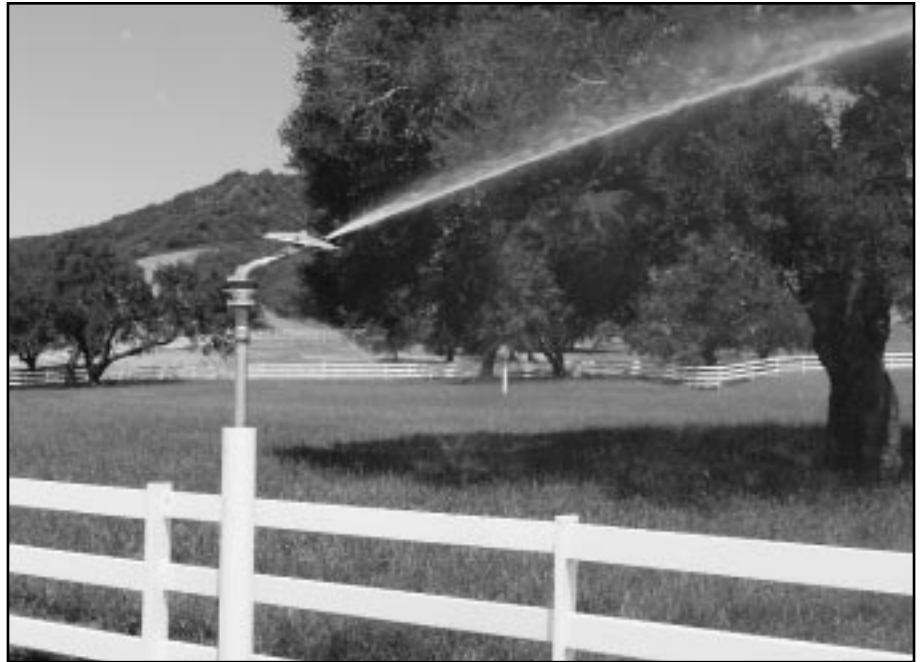
Controlling a Rain Bird Rain Gun on a remote pasture without electric power or wiring.
