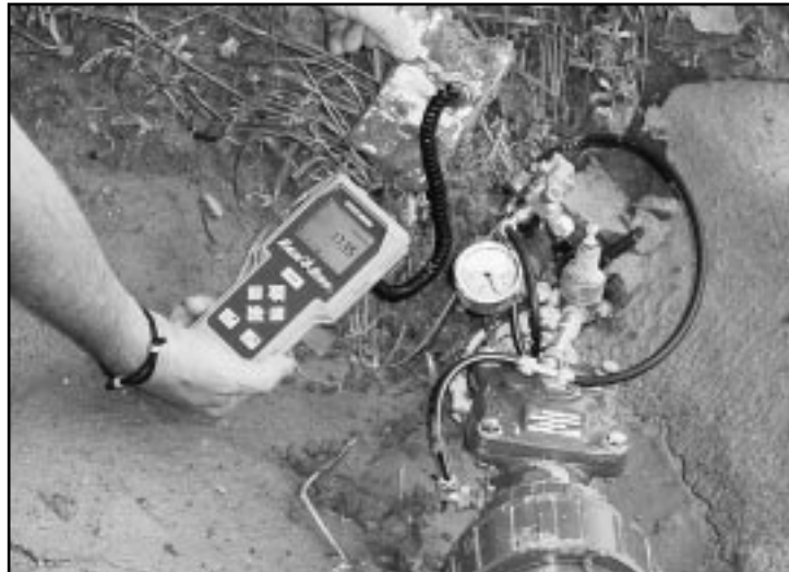
This control module and valve were buried for 2 weeks due to flooding. Infra-red communication with the field transmitter still worked.
